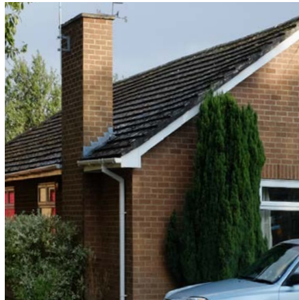
Brick tends to be treated simply, without complicated detailing or patterns. Bricks in white, yellow, buff and red are used throughout.
